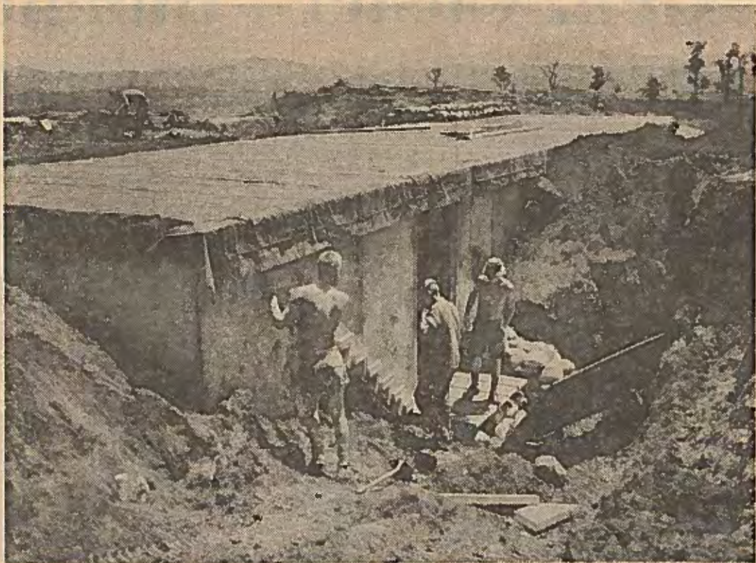
Seabees install a stairway into one of the buildings being built at the Con Thien Special Forces camp. Much of the camp is being built underground.
